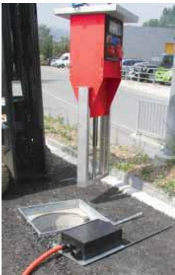
Prepared cable connection box with flexible supply line to the underfloor distributor.
