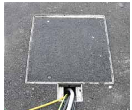
Filling up the reservoir cover with asphalt, match up the environment using the same filler material and adjust the height to the upper reservoir part.
