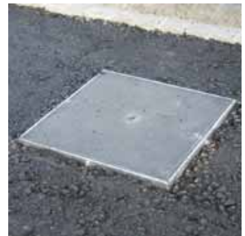
Fill in the frame with asphalt to install the fine layer. Final layer follows later on.
