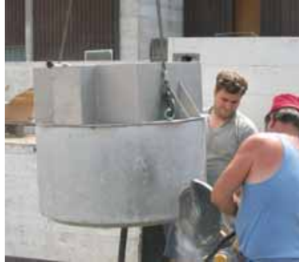
The standard concrete tube included and pre-mounted with the stainless steel construction is prepared for installation: Milling out an opening for the supply cable.
