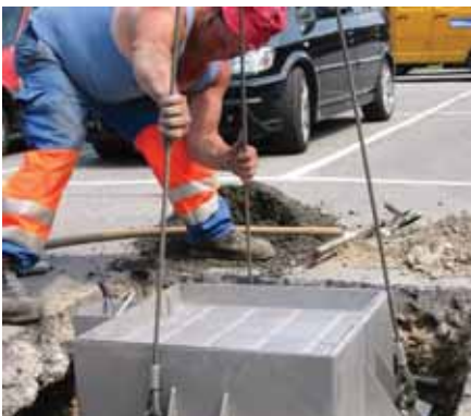
Fit the unit and level off to the correct installation depth (level with asphalt).
