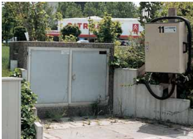
Plastic terminal box (Power station, Weinfelden)
