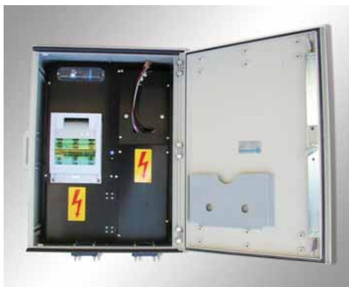
NIV terminal box 300 A in plastic distribution box 600x800 mm (Services Industriels, Lausanne)
