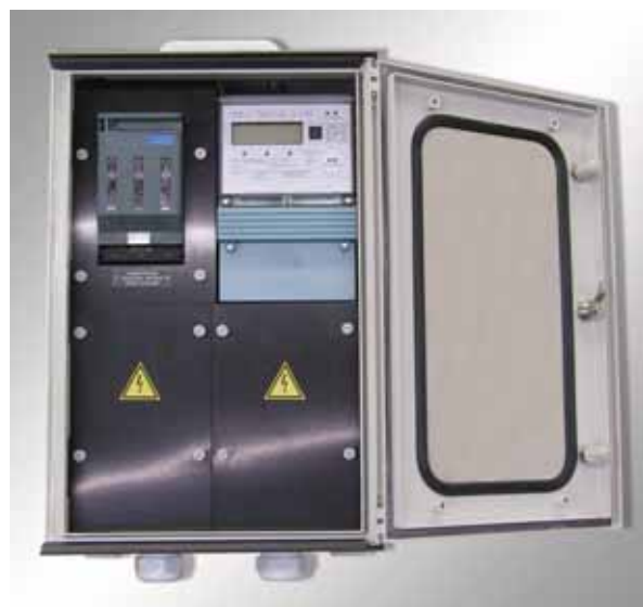
NIV terminal box, 100 A in plastic cabinet 400x600 mm with viewing window (Romande Energie SA)
