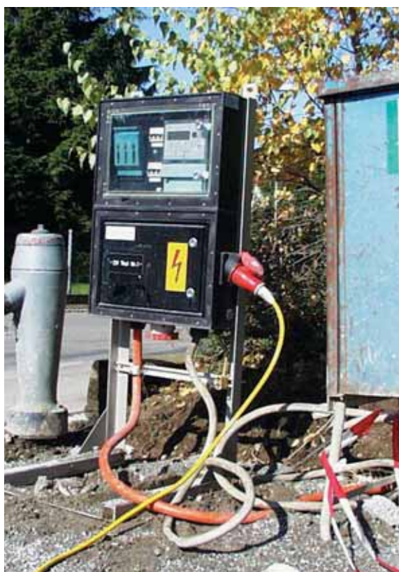
NIV terminal box 125 A (Power station, Thal)
