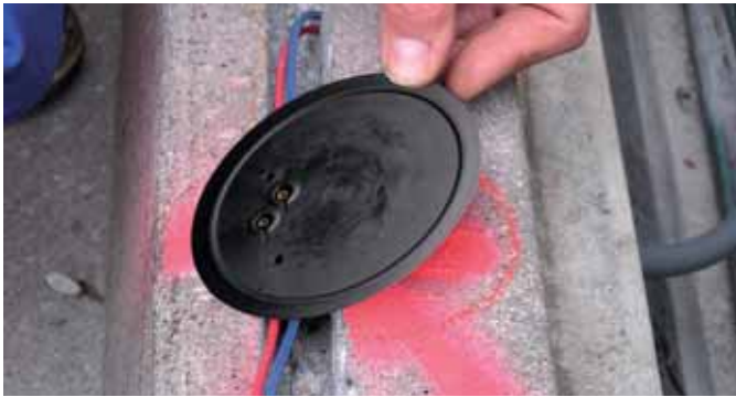
Installation of current collector on flexible wires
