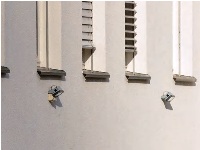
SpotLED 230 as outside illumination of municipal buildings
