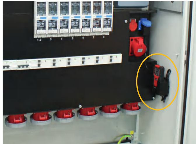
TorchLED Emergency in a construction site cabinet
