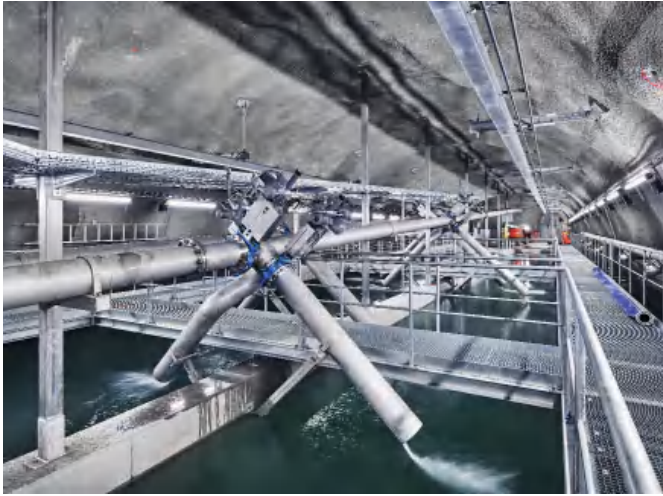
StreamLED 2: Customer / installation engineer: BLS Netz AG EPRO TRAFFIC GmbH: Electrical engineer
